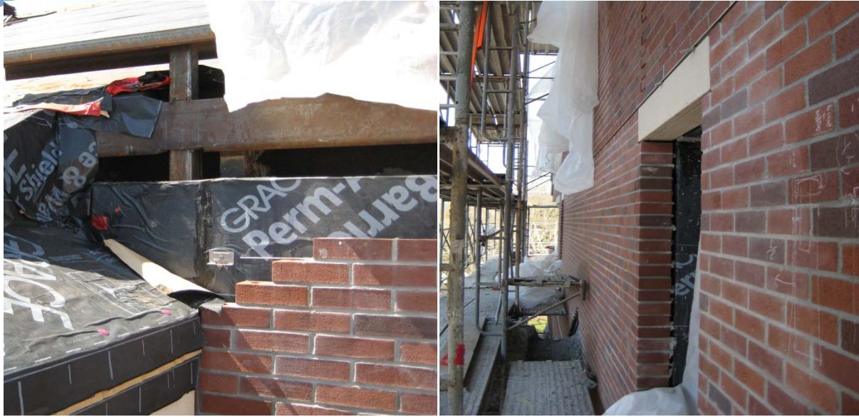
The two images above were taken of the full size brick façade during construction of the SRJC Student Center
